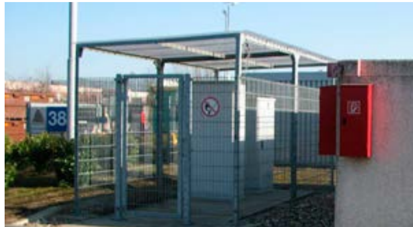
Figure 4.14: Fuel cell UPS installation (source: Aluminium Norf GmbH)
